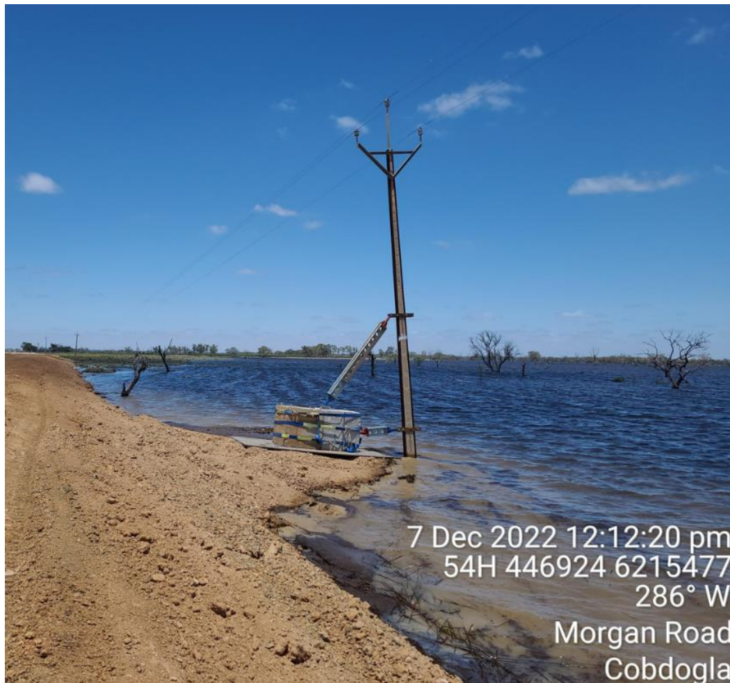
Figure 9 - Pole with temporary support to prevent failure.
