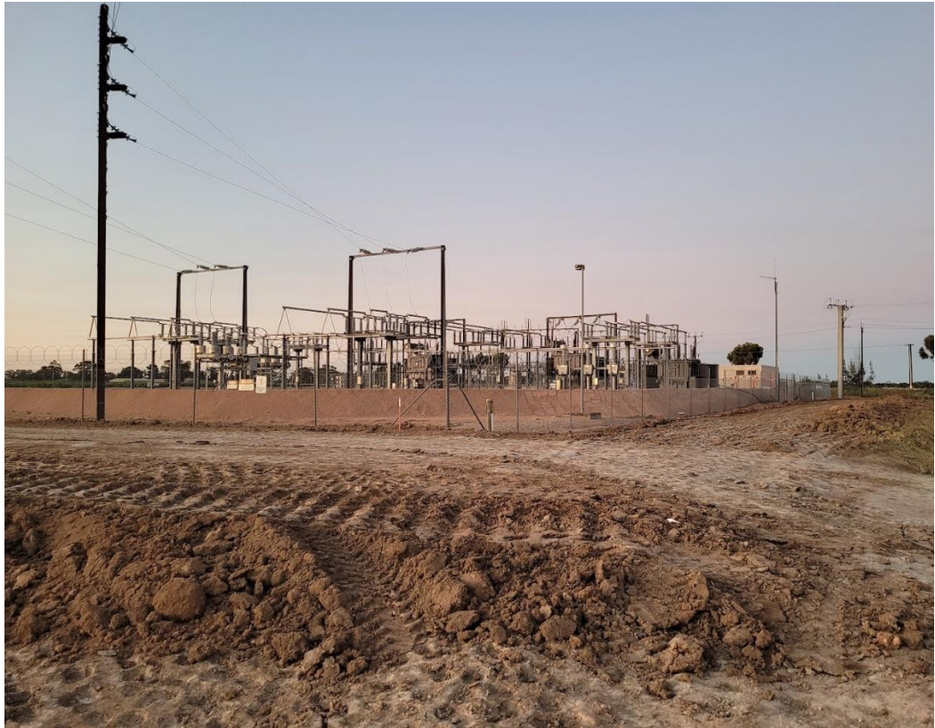
Figure 11 – photo of the two bunds/levees protecting Renmark zone substation.
