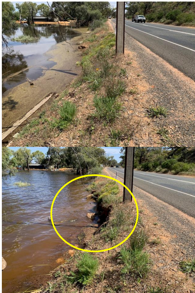
Figure 8 - Impact of flood water on pole footing.
