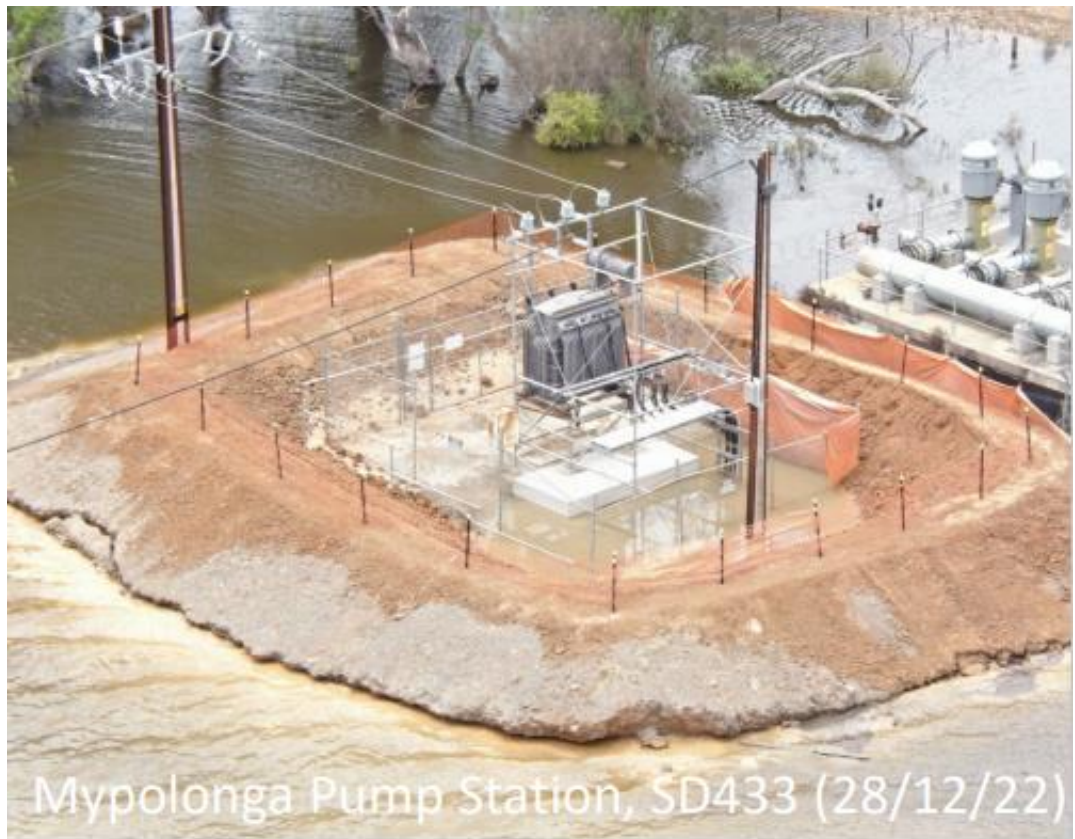
Figure 12 - Bunding around the Mypolonga transformer station, which supplies the pumping station.
