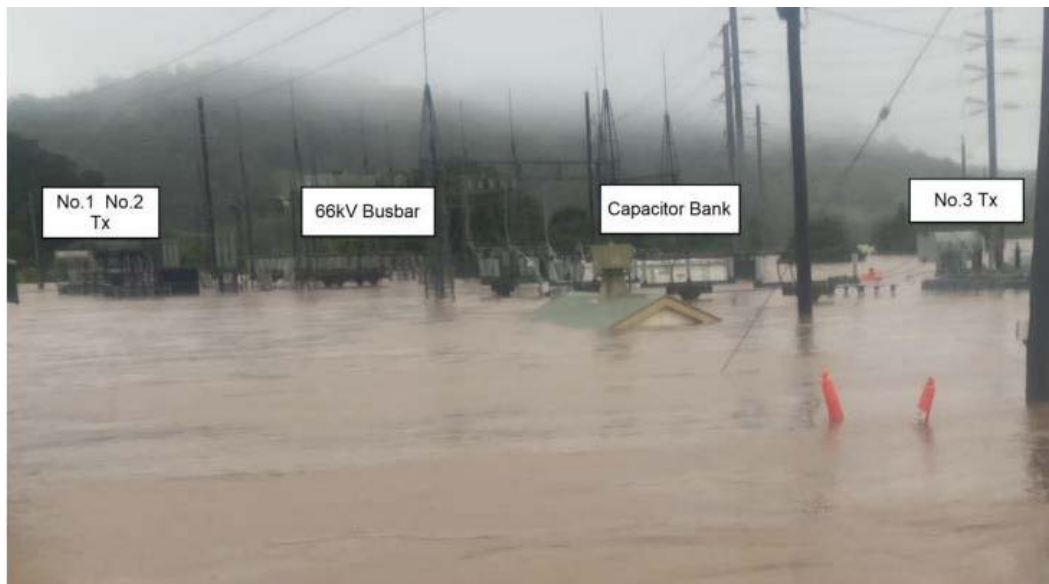
Figure 4.6: South Lismore zone substation 28 th February 2022
