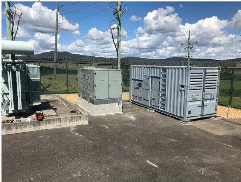
Figure 4.4: Urbenville microgrid project
