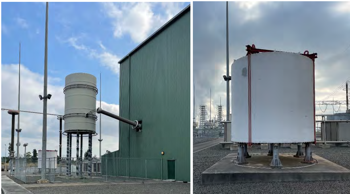
Figure 7.4 Basslink's smoothing reactors
