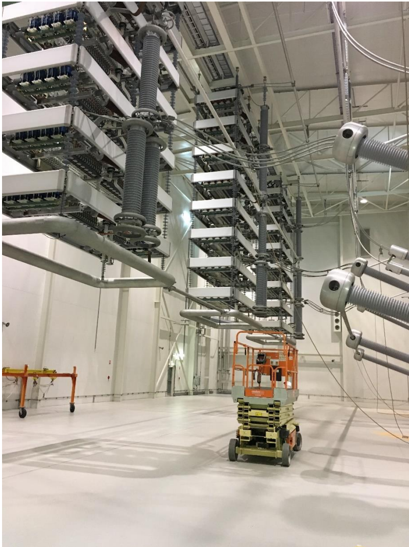
Figure 2.2 Basslink's Thyristor Valve Hall
