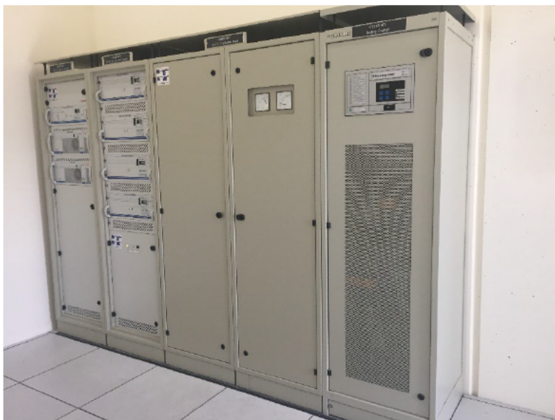
Figure 13. DC Distribution and Charger Overview
