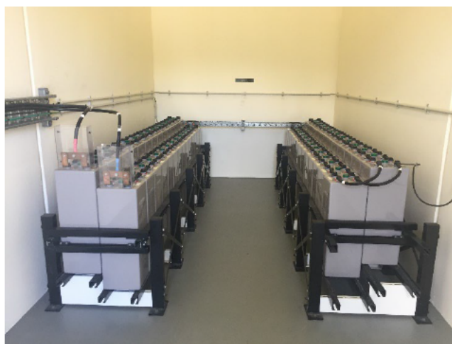
Figure 14. 110V Battery Overview
