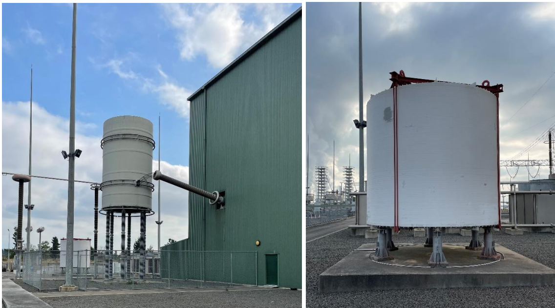
Figure 7.4 Basslink's smoothing reactors
